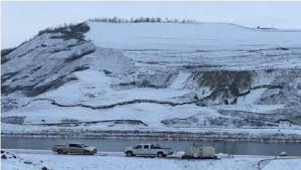
Picture X 4 CBC Feb 24, 2017 a 400 meter long crack appeared during construction activities.
