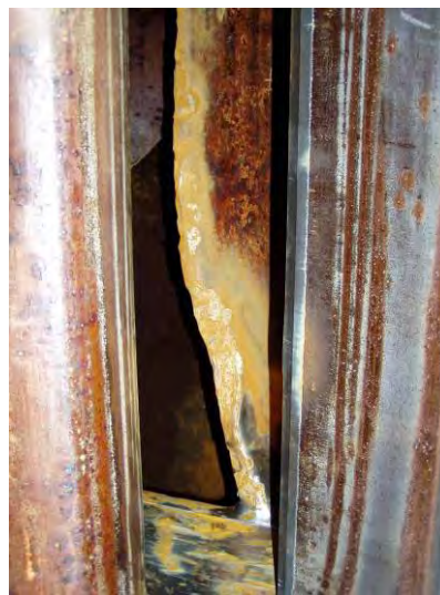
Figure 9: Moderately Damaged Inlet Edge
