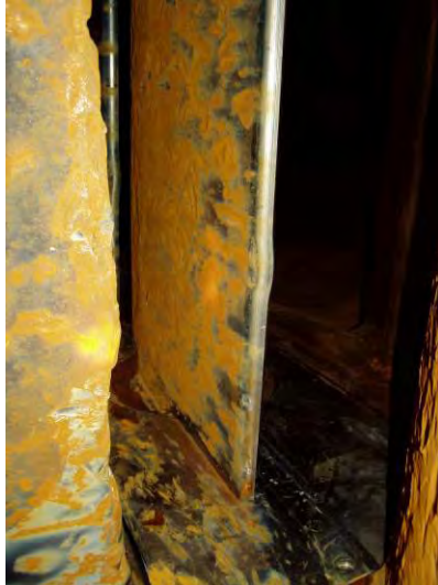
Figure 4: Wicket Gate Trailing Edge Damage
