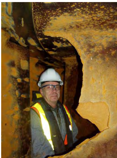
Figure 8: Severely Damaged Inlet Edge
