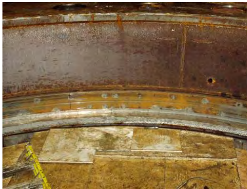
Figure 11: Carbon Steel Deposited on Lower Seal Ring
