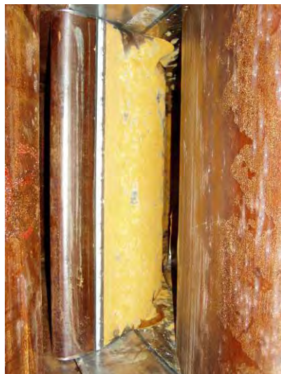
Figure 2: Wicket Gate Skin Plate Damage
