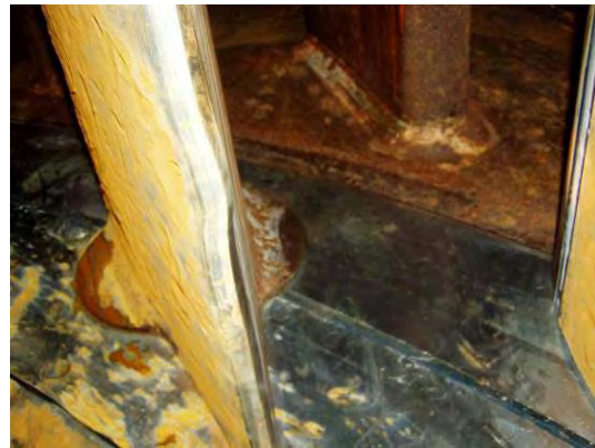
Figure 5: Wicket Gate Trailing Edge Damage
