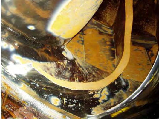
Figure 6: Missing Blade Piece
