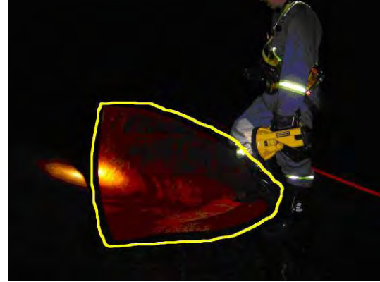
Figure 7: Missing Blade Piece Found in Draft Tube
