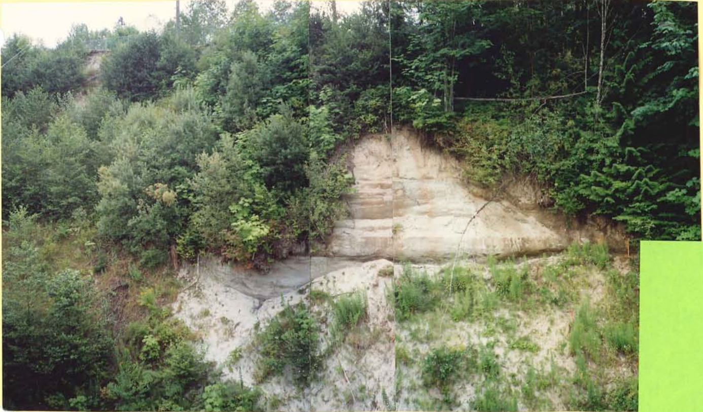
Photo 13 - Slope above Unit 3 before stabilization work.
