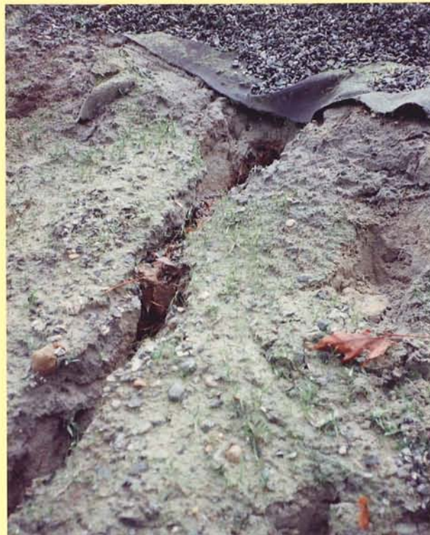
Photo 16 - Erosion observed at location of arrow on Photo 15.
