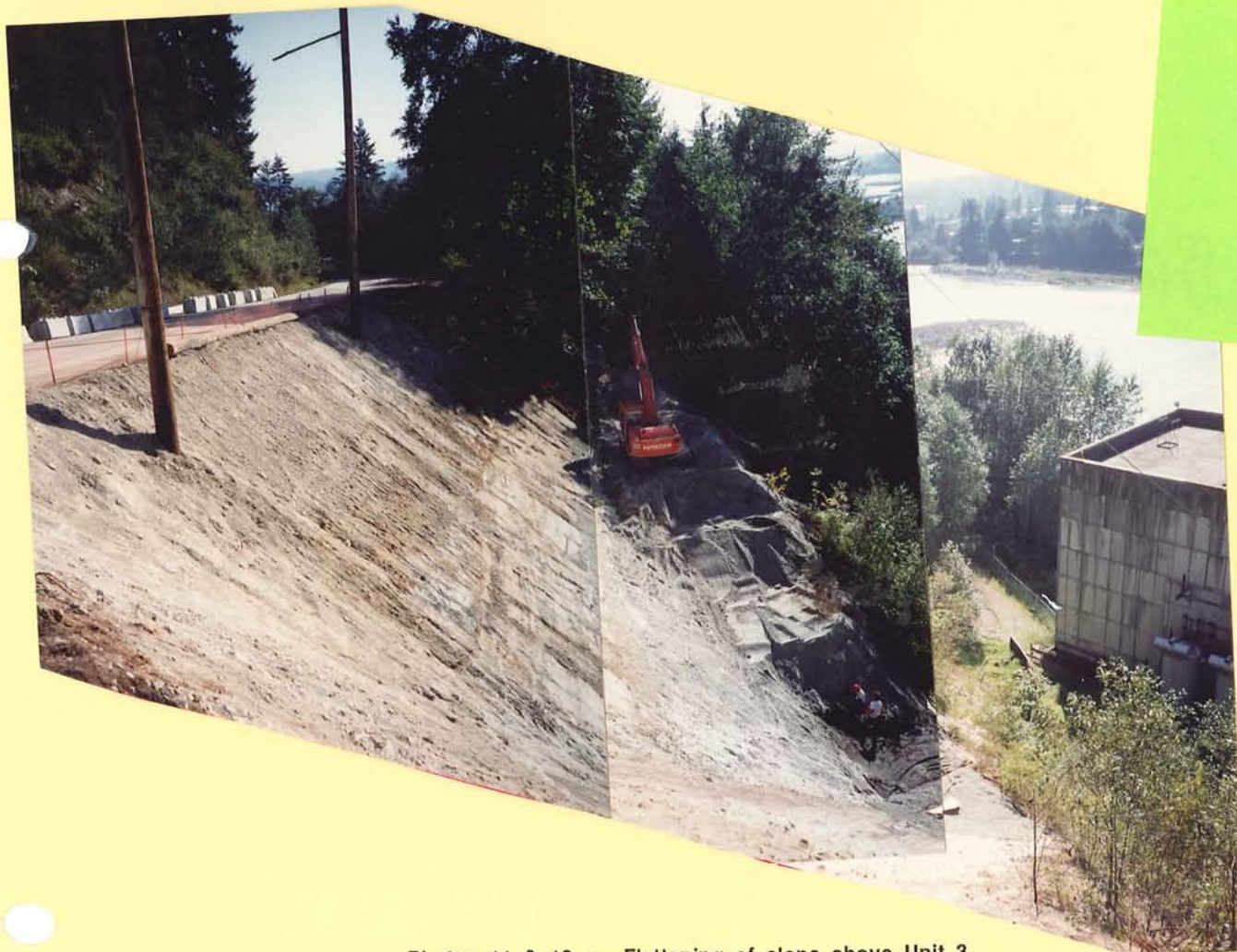
Photos 11 & 12 - Flattening of slope above Unit 3
